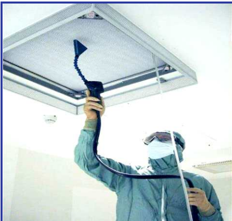
HEPA Filter Integrity / Leak Testing
