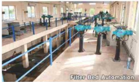
Filter Bed Automation
