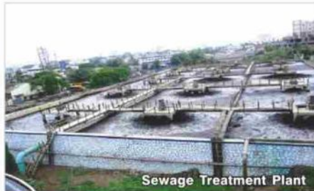
Sewage Treatment Plant
